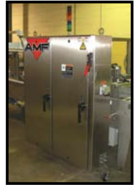
Machine Mounted Electrical Panel
